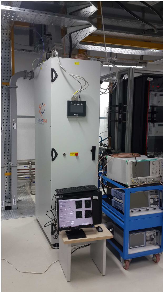
Figure 8: Photo of TARLA 1.3 GHz RF amplifiers with test setup.
