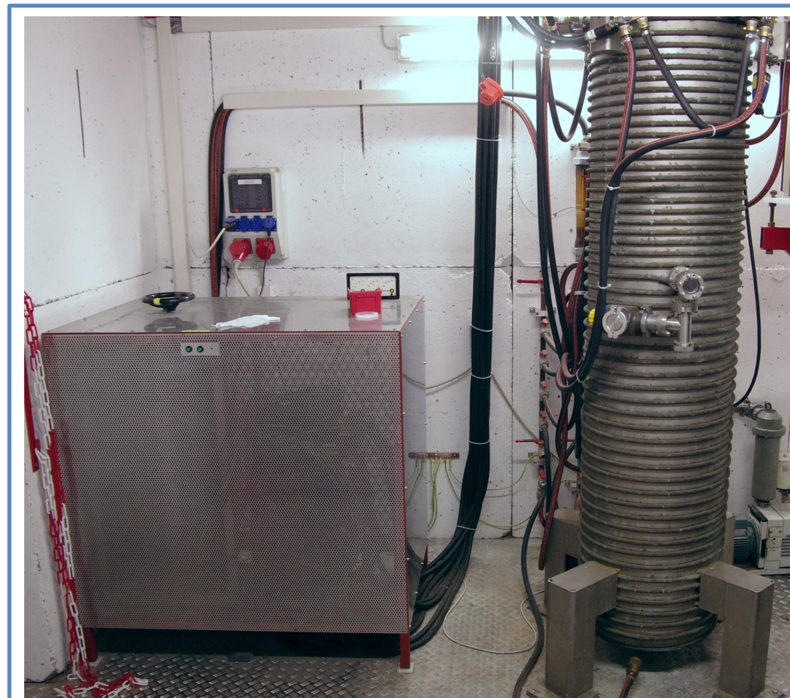
Power supply and furnace
