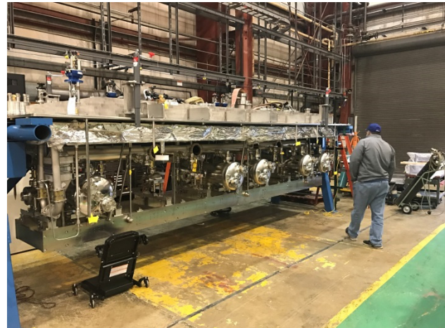
Figure 5: The HWR cold-mass hanging from the lid prior to installing on the lower vacuum vessel. This was a “mock” assembly to practice for the final assembly and to verify that the components go together.
