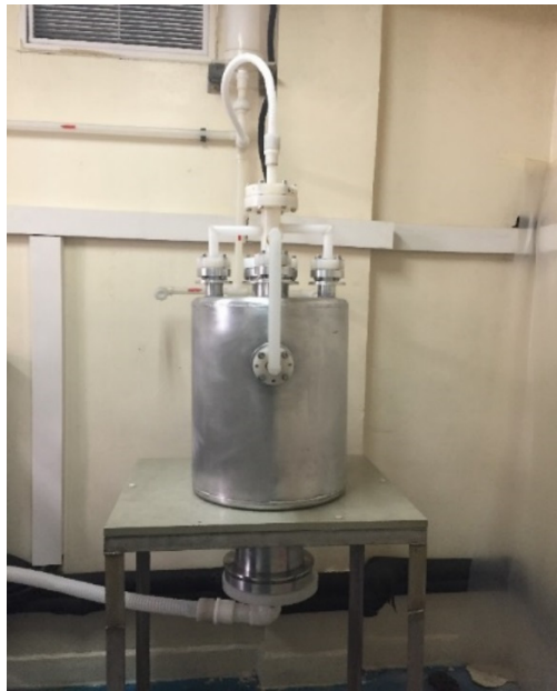
Figure 2: Buffered chemical polishing system.
