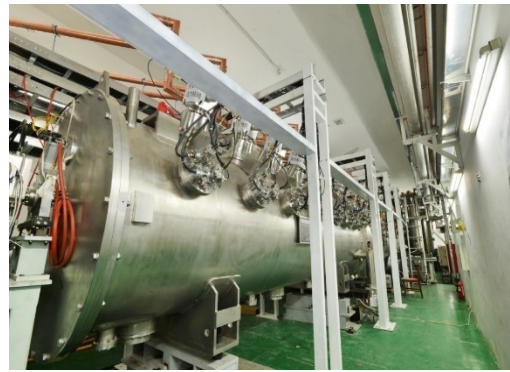
Figure 5: The two cryomodules of Injector-I installed in the tunnel.
