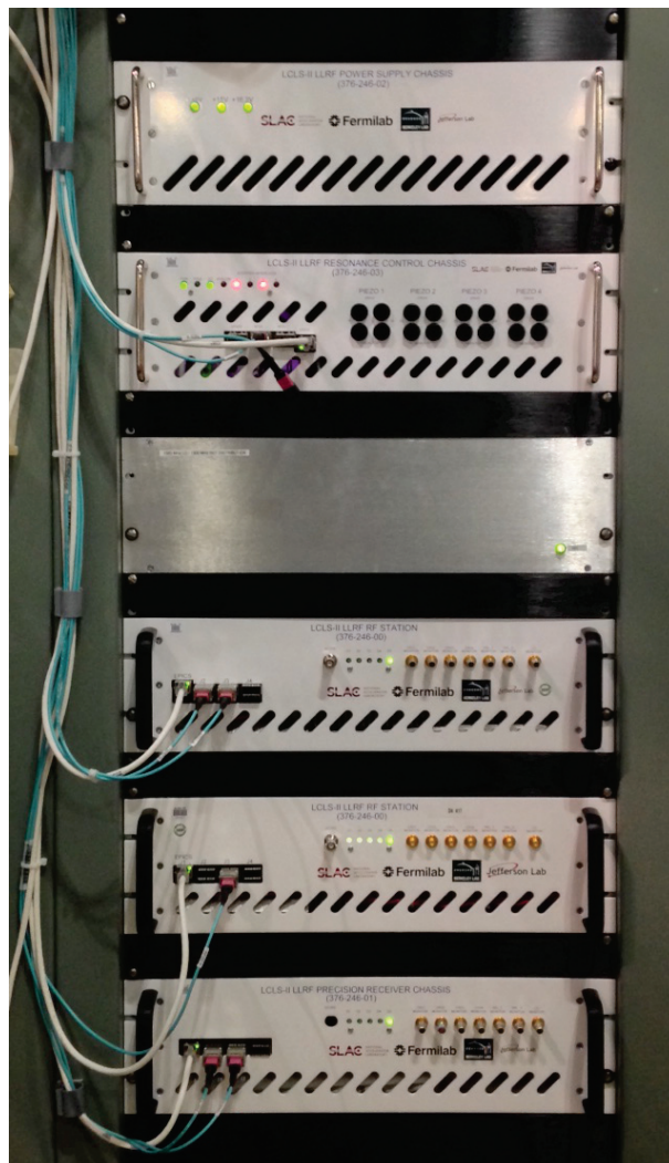
Figure 11: Prototype Chassis installed at the FNAL CMTS.
