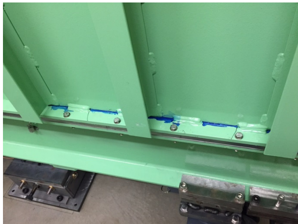
Figure 13: Vacuum leak location of the SCM501 cryomodule vacuum cover. Leak location was vessel welding defect.
