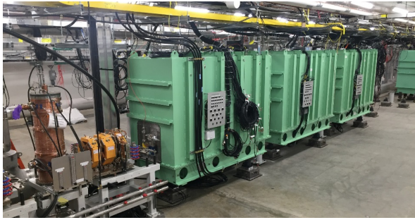
Figure 11: Installed 0.041 three cryomodules in the FRIB tunnel.
