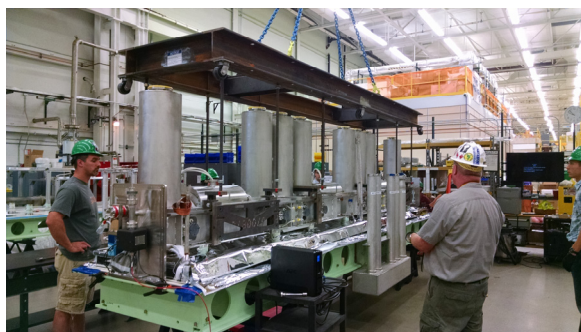
Figure 3: Coldmass mounting on the cryomodule baseplate.
