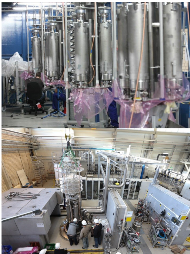
Figure 1: Preparation area for vertical testing (top) and vertical test installations (bottom) at AMTF.
