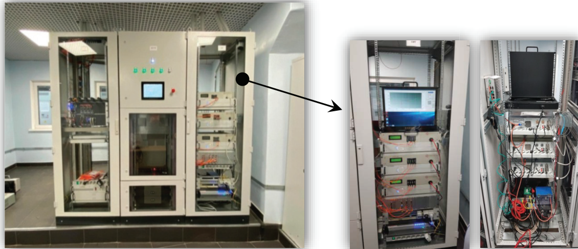
general view of the measuring equipment
