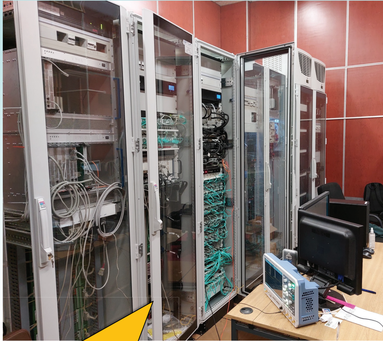
New control system racks
