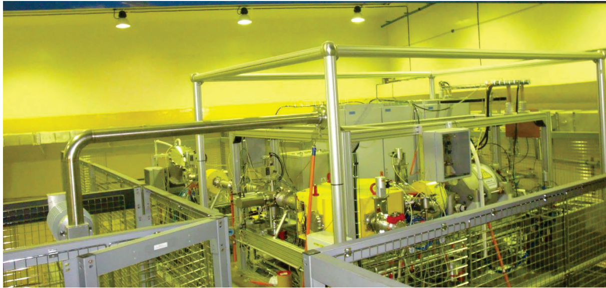
The HV platform
