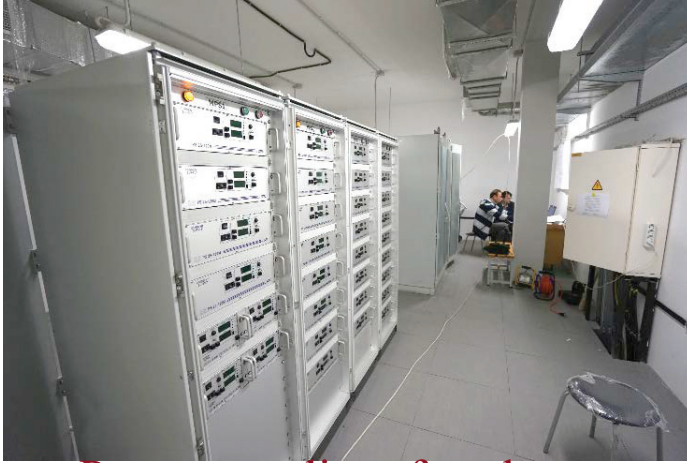
Power supplies of cyclotron
