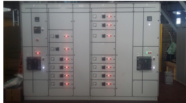
Figure 2: Main electrical rack.
