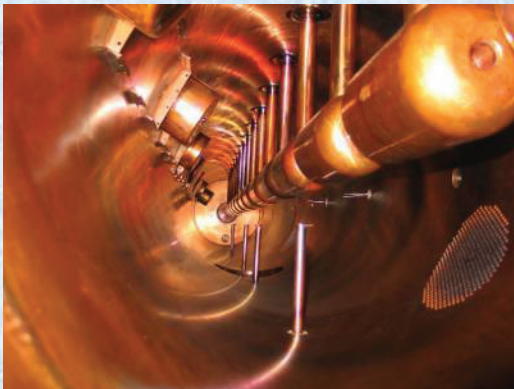
Inside Drift Tube Tank
