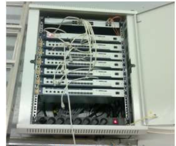
Rack after the installation of electronics units
