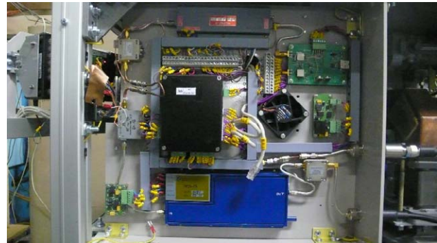
Figure 7: RF and cooling system controller.
