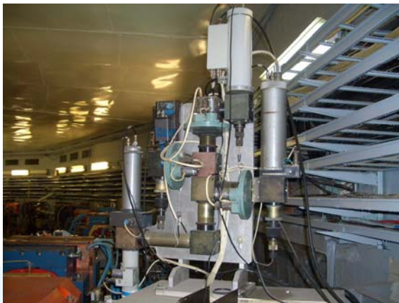
Existed optical system of electron beam observation inside of tunnel of SIBERIA-2
