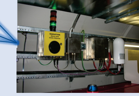
Radiation + Alarm Units
