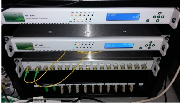
Figure 2: Installation of the GFT 3001 Master Oscillator and GFT 1004 Digital Delay Generator in Oscillator Room 2.
