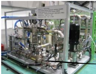
Fabricated water pumping skip
