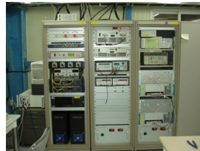
LLRF Control System
