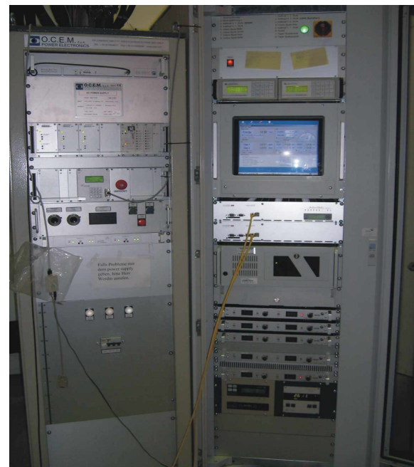
Figure 4: Updated SCU14 control system. On the right, the temperature controller, both UIOCs, five corrector power supplies and the TPG-vacuum controller can be
