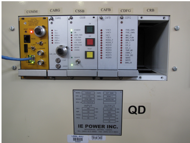
Figure 2: DPSC Installation at Booster QD Power Supply (far left).
