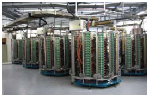
Figure 2: Amplifiers 1 and 2 in the SR RF room.
