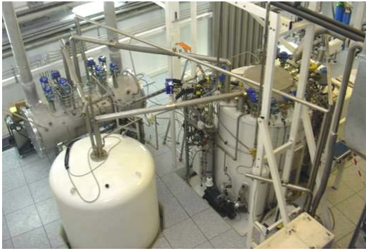
Figure 4: The cryogenic area in the technical gallery.
