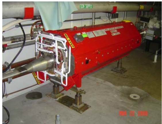
Figure 3: A WQB installed at the Q222 location.
