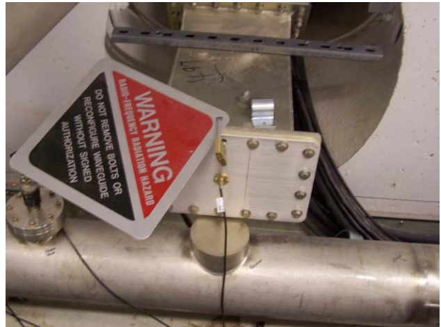
Figure 3: Waveguide Flange Locked Out
