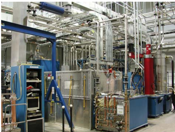
Figure. 1: The layout of the high power RF system in the RFTF.
