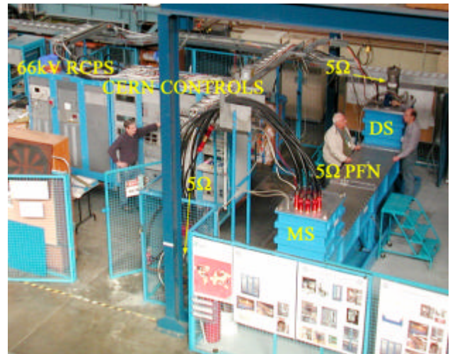
Figure 1: High Voltage Test Setup at TRIUMF.
