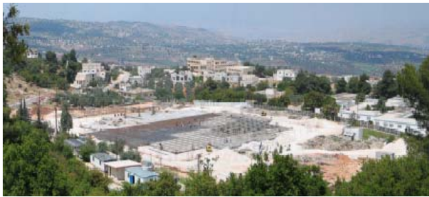
Figure 1: A panoramic view of SESAME building during construction (April 2005). In the picture is clearly visible the floor of the experimental hall.
