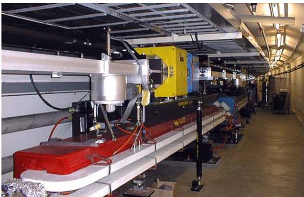
Figure 1. View of the PEP-II tunnel.
