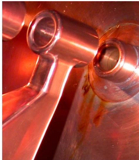
Figure 1. Soldering flux patch in DTL tank #4
