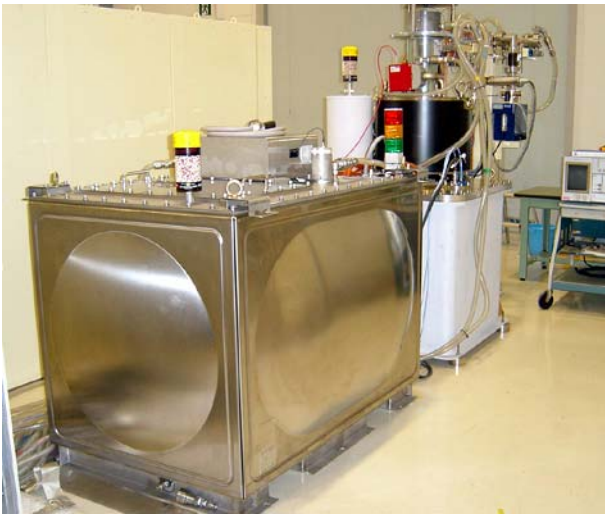
Figure 4: Klystron modulator (front) and 50 MW C-band klystron with pulse transformer tank (back).
