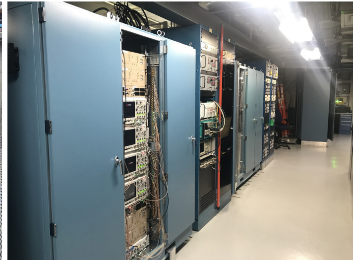
Pulsed Power Units installed at FXR
