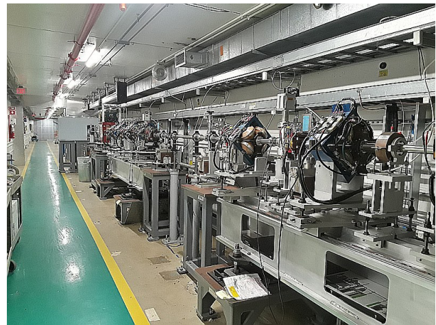
Figure 3: Photograph of the installed LEA beamline.
