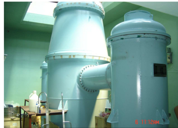
ELV-12 BINP with EB Tech; 1 MeV, 400 kW
