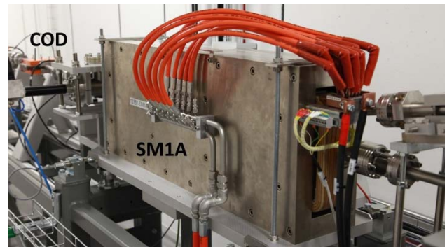
Figure 5: The septum magnets 7 are Lambertson type, bending the beam upward from the linac into the transfer lines (SM1A, SM3A), and downward to emerge parallel with stored beam in the rings (SM1B, SM3B). This photo is from Solaris 2015, where SM1A is used simply as a bending magnet. At MAX IV, SM1A and SM3A are each preceded by a pair of dipoles (DIH) shifting the beam sideways into the septum pole gap, selecting if the beam is taken up into the transfer line or straight through the septum channel.
