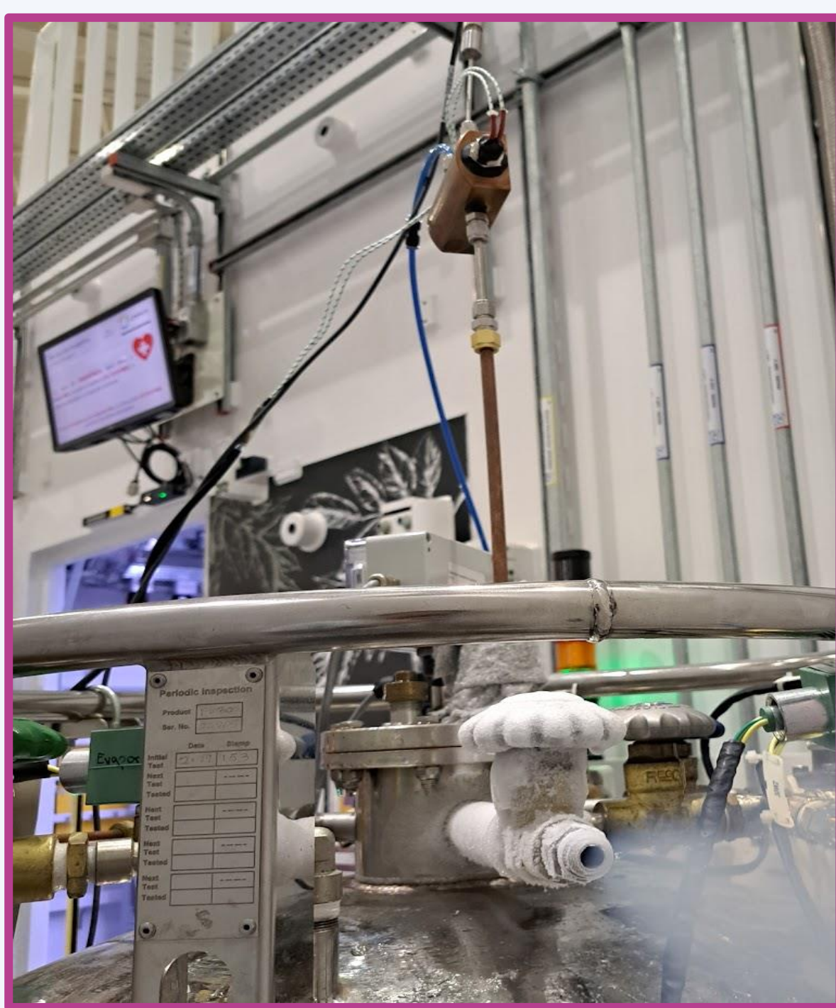
Hot gN2 purging process.
