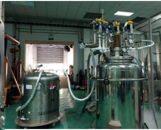
Cryo Cooling System
