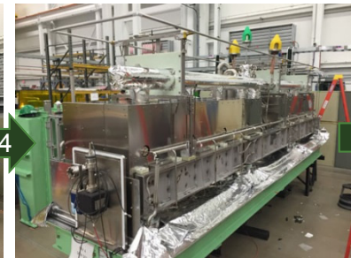
Completed cryogenic circuit
