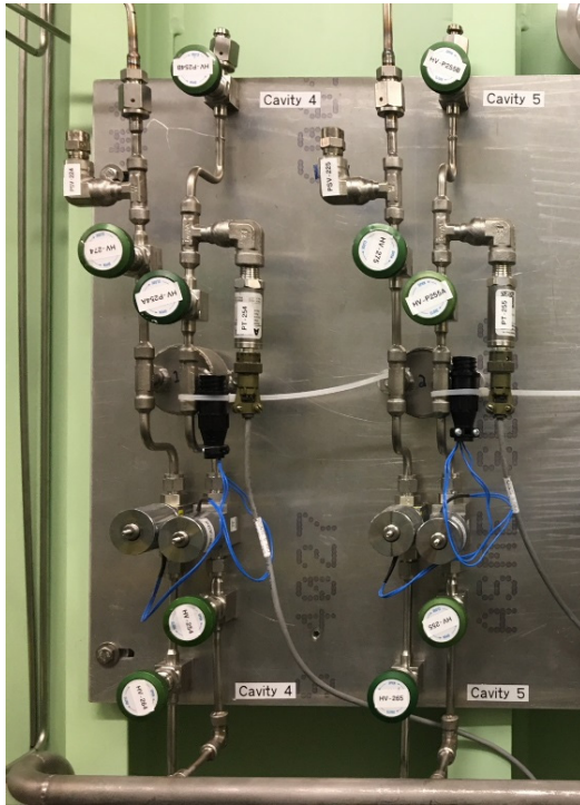
Manual valves on pneumatic tuner gas distribution manifold
