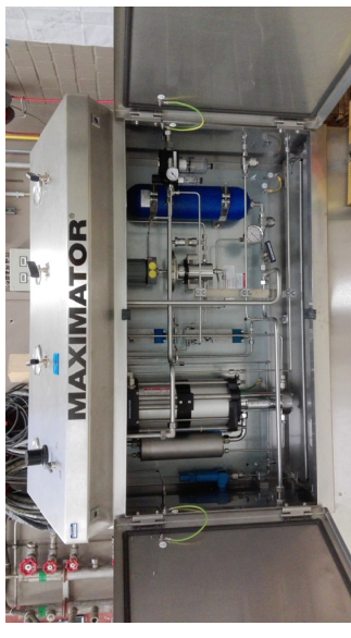
High pressure hydrogen compressor (ATEX, 600 bar)
