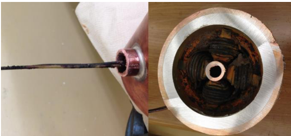
Figure 11: Enamel coating separation from the wire (left) and the yoke covered with rust (right).
