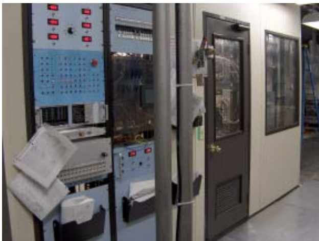
Figure 5: HV power supply.
