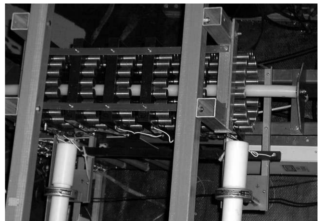
Figure 1: 60Kv 20A-50A switch as installed at the base of the IPNS ion source.
