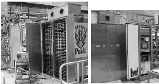
Figure 1: "8-pack" Solid State modulator installation.
