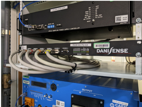
Figure 2: System hardware installed in P.S. cabinet.
