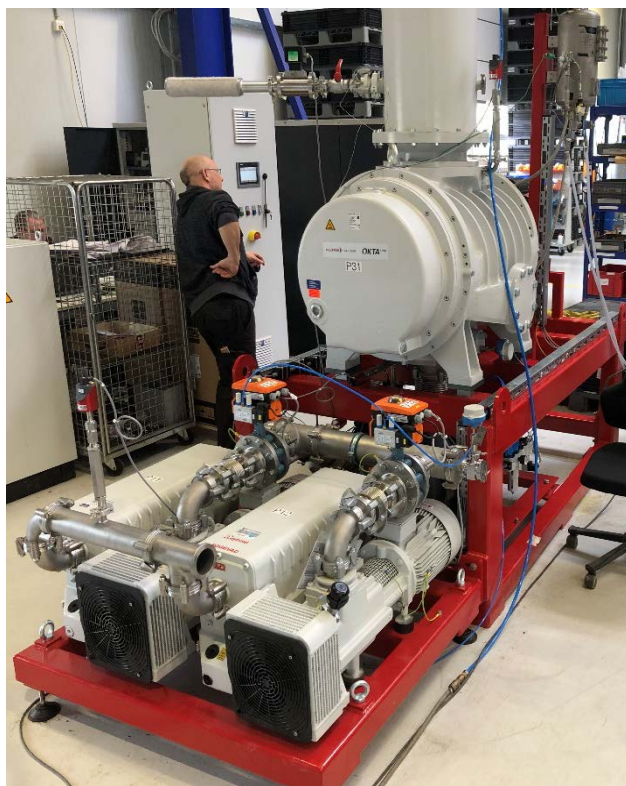
Figure 8: Photo of the ATEX roots pumping station during the Factory Acceptance Test FAT at Pfeiffer, Aßlar.
