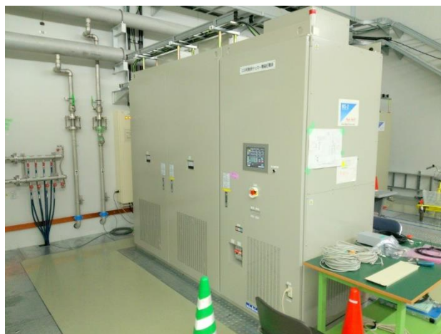
Power supply (60 Hz, 1 kV-299 A)
