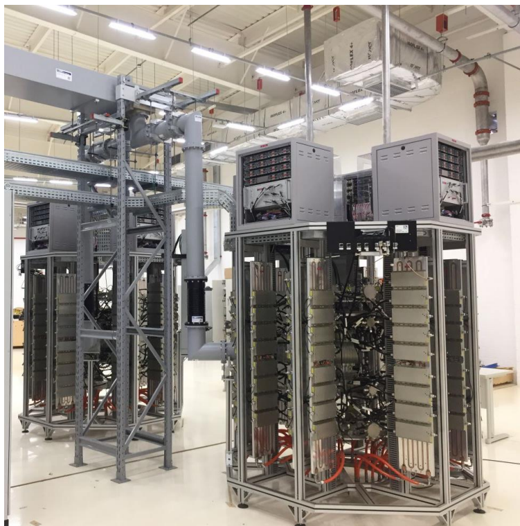
Two 60 kW RF amplifiers installed at the RF Room
