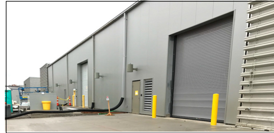
Figure 7: The PPU portion of the klystron gallery with new pump room in the foreground and new exterior electrical switchgear in the background along the previously existing klystron gallery.
