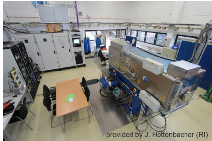
Figure 2: Test stand for factory acceptance tests of the cavity and amplifiers at RI (courtesy of RI Research Instruments GmbH).
