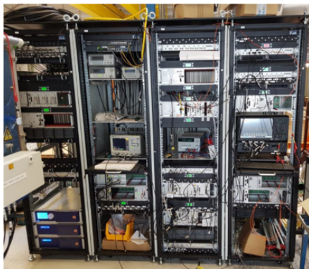
Figure 6: Installation of the LLRF racks in the test stand of the AC first of series RF station at GSI.
