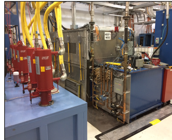
AT HVC under going heat test
