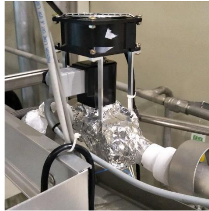
Figure 11: After install protection instrument, there is no condensed water or frost surround the relief valve (foil covered) at \text{LN}_2 refilling period.
