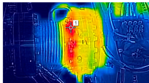
Figure 2: Thermal image of the attached bellows to the flange of the vacuum chamber made by the FLIR AX8 infrared camera, where the local overheating appeared.
